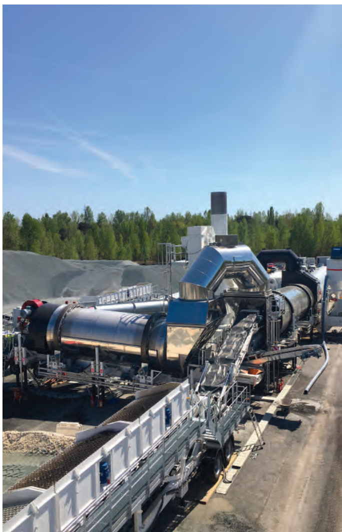
The Ermont TRX Highway asphalt plant: up to 100% Reclaimed Asphalt Pavement (RAP)
