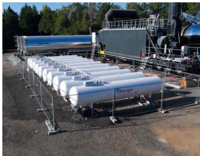
LPG storage for Ermont asphalt plant
