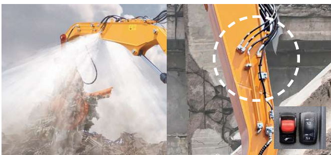
Water Spray Nozzle installed (Total 4 ea)
