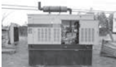
1998 CAT GENERATOR , stk# 223-15, s/n 98A-02737-S
