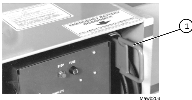
Figure 2-2. 350 Amp Battery Connectors
