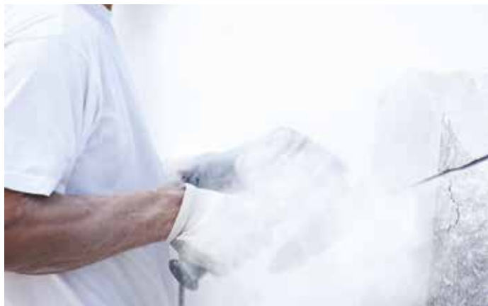
Silica dust is generated in workplace mechanical processes such as crushing, cutting, drilling, grinding, sawing or polishing of natural stone or man-made products that contain silica
